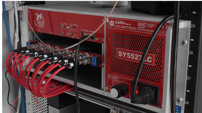
Figure 3.11: Picture of the multichannel HV power supply system.
