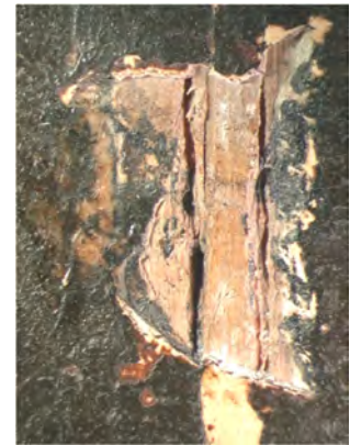
Abb. 3.2.6 / 9 (B_IV_09) Brett V/a Bohrlochschaden; Lokal. ↑ 31,7 - 33,0 cm → 4,0 - 5,0 cm
