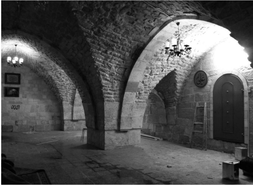
Fig. 8 – Section of the hall in the northwest, today part of the Omar Mosque (photo: Jürgen Krüger, 2011).
