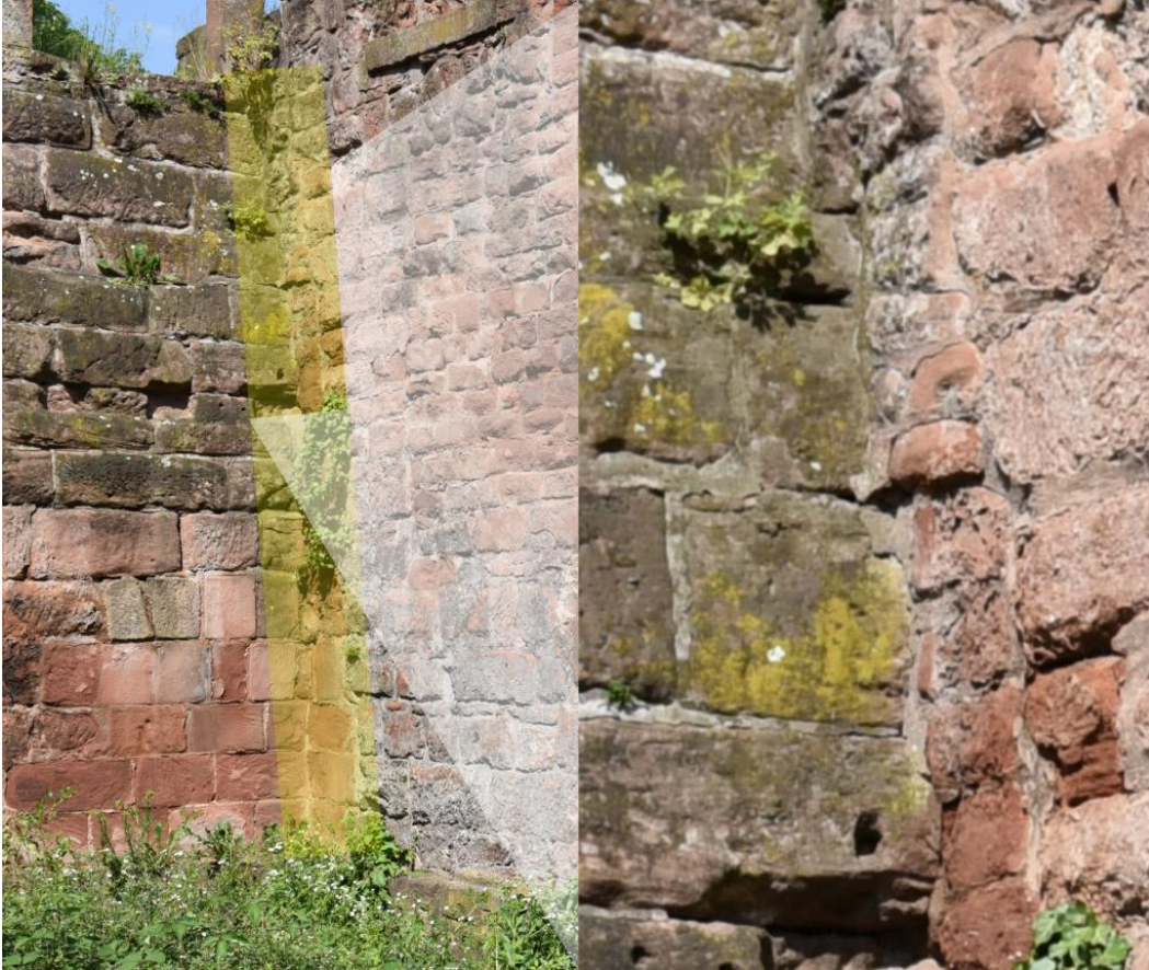
Figure 28: Connection of the western section of Inner Chamber D to the eastern Curtain Wall with close up (right).
