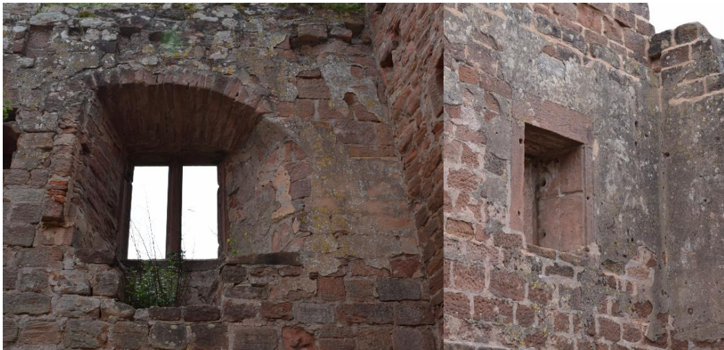
Figure 61: Plaster to around Window 3 (left) in Chamber A and Window 5 (right) in Chamber C.
