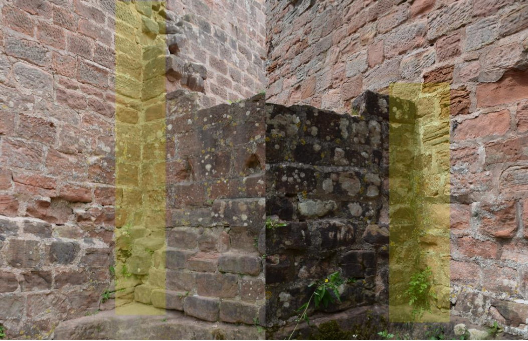
Figure 60: Middle basement wall of Inner Chamber C connected to the southern (left) and northern (right) walls.
