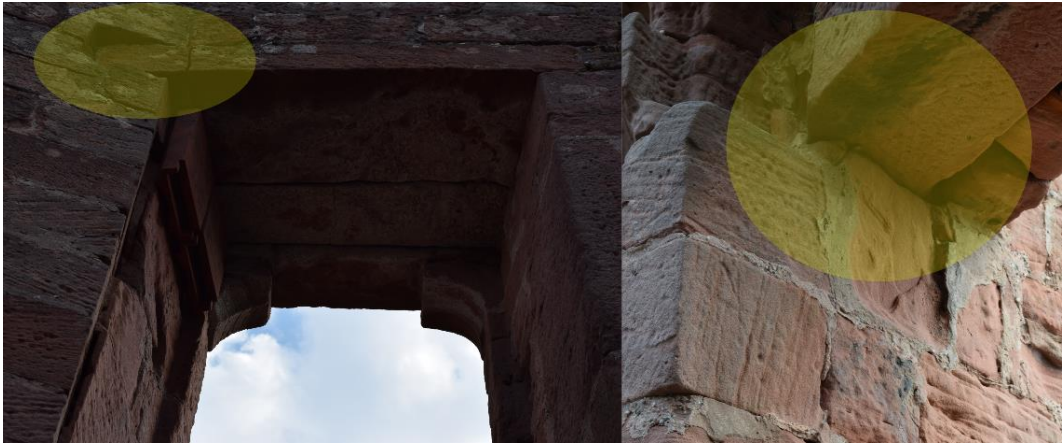
Figure 58: Interlocking lintels of Portals 2 and 3 with the southwestern edge of Inner Chamber C.
