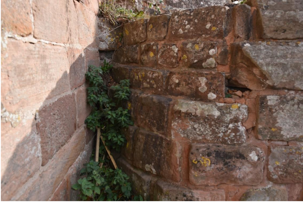
Figure 52: Connection of the main tower (right) to the shield wall (left). Note the difference in masonry styles clearly indicating different building phases and, likely, different masons.
