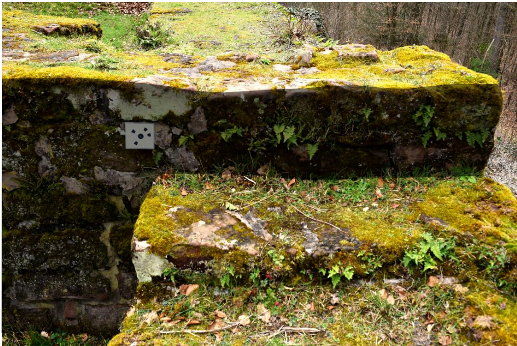
Figure 65: Connection of the northern end of the separating wall and the outer wall.
