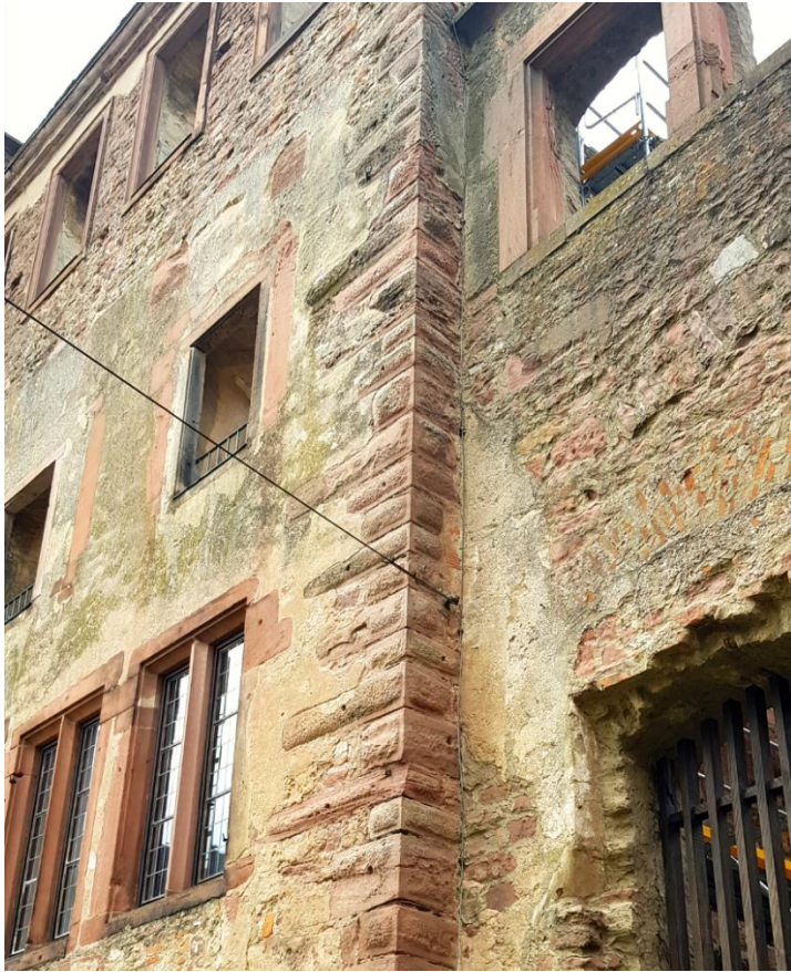
Figure 40: 15 th century windows (top left) at Heidelberg castle next to embossed quoins.
