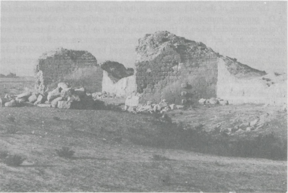
Fig. 4. Two stone bastions built against the original mudbrick wall. (Photo by M. Gawlikowski)
