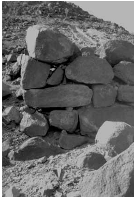
Fig. 32. Unstable stone frame of the bastion after erosion of the clay mortar.
