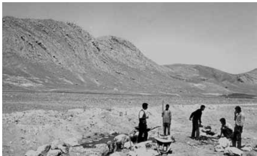
Fig. 30. Labourers building a house. The stones are packed individually in clay before the next layer is laid (stone-in-clay building method).
