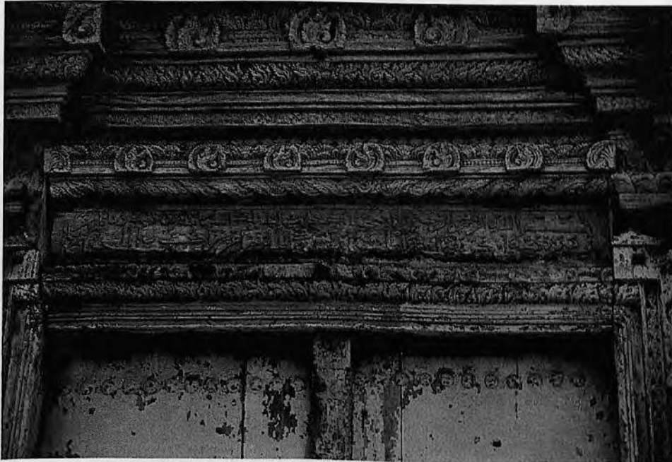
Pl. 10 Lintel of the front door of the house of the wālī of Bawshar (P.Y.)
