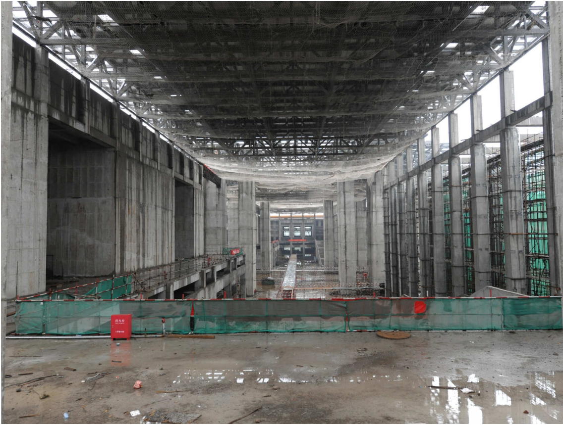
Figure 13: National Museum of China, Grand Forum under construction, courtesy of Dong Qing, June 2009
