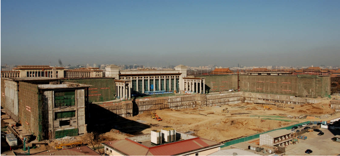
Figure 11: National Museum of China, construction site from the east, courtesy of Dong Qing, Feb.2008
