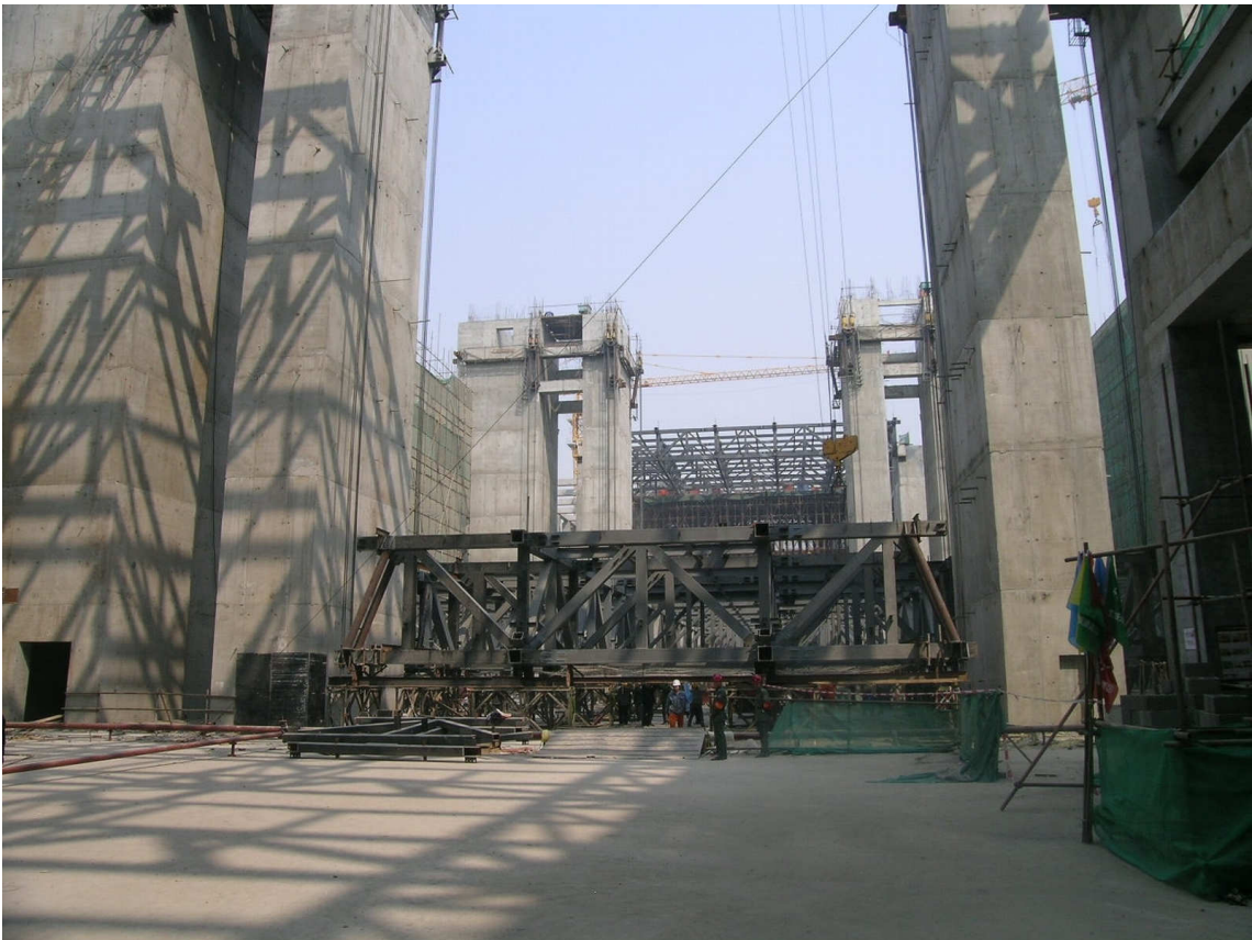
Figure 12: National Museum of China, Grand Forum, raising of the bearing structure, March 2009
