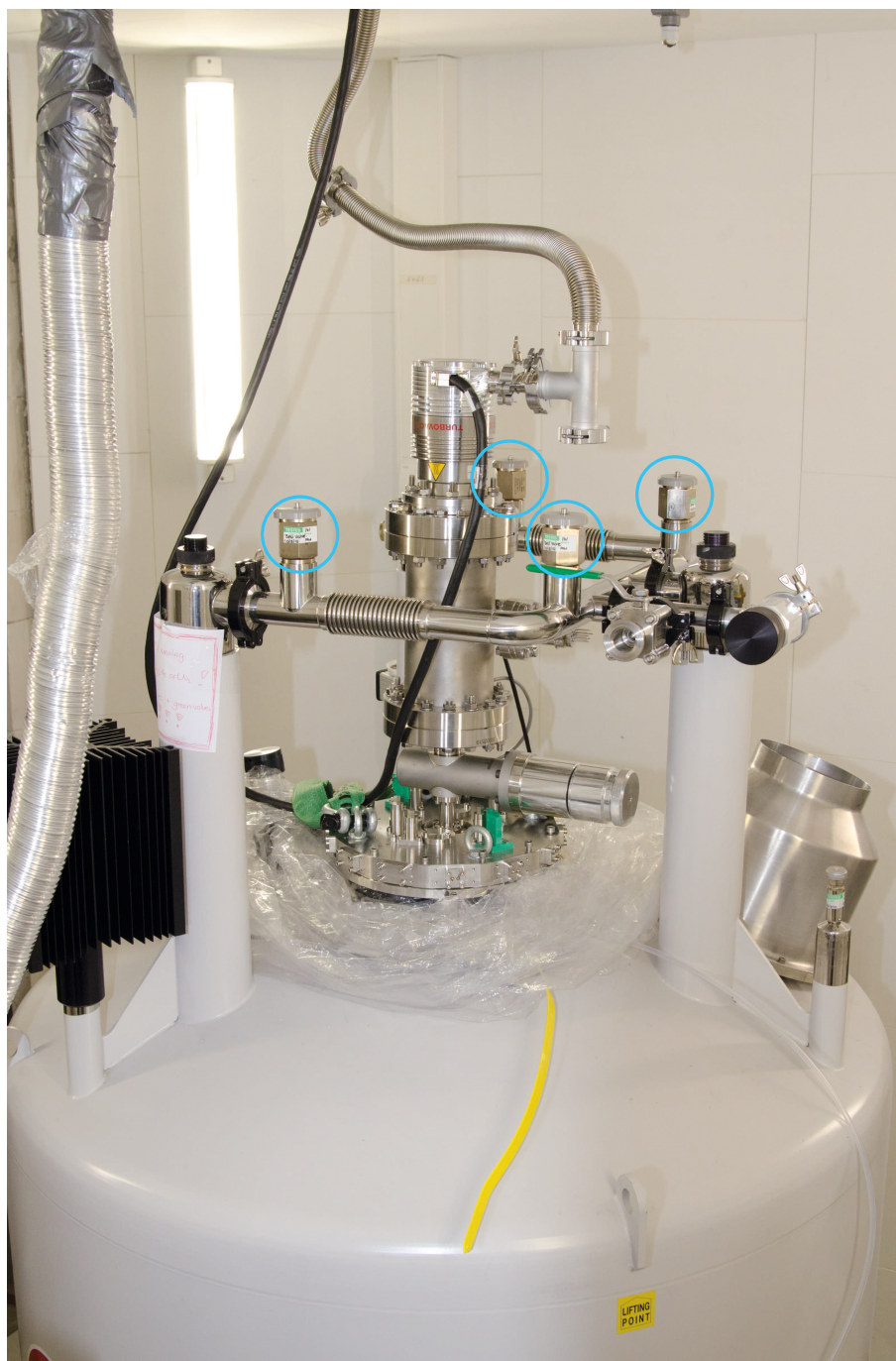
Figure A.3: PENTATRAP magnet with safety valves indicated in blue. These valves open at an overpressure of about 200 mbar.
