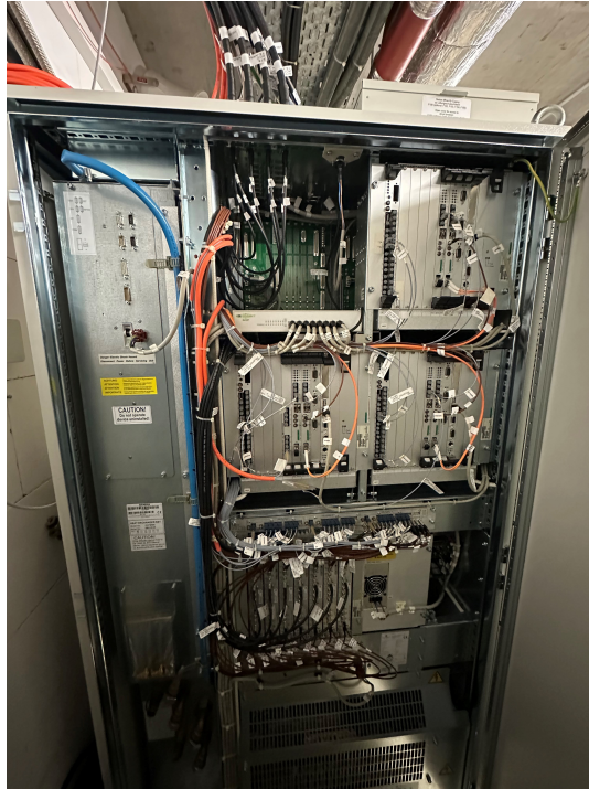
Figure 9: Photograph of the Siemens pTx system "Step 2.3".
