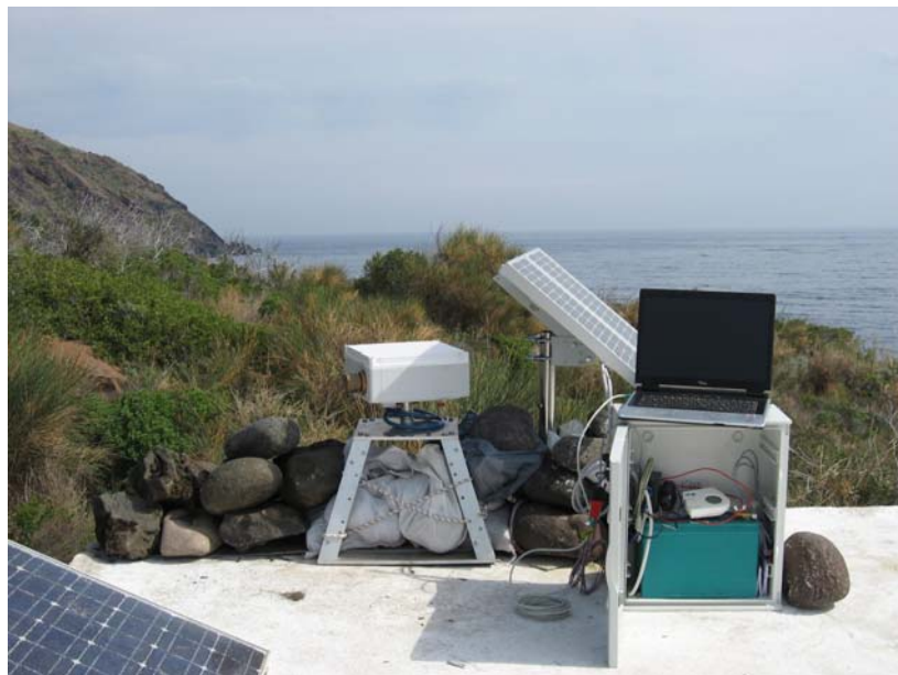
Fig. 5.6 – Installation at Punta Lena. The NOVA mark II instrument is mounted on an aluminum structure on the roof of a small building. It is weighed down by stones. An additional housing contains the 100 Ah solar battery, which in turn is charged by a solar panel. The instrument is switched off at night with a 12V DC timer. The laptop computer is not part of the installation, but is only used to download data from the instrument.
