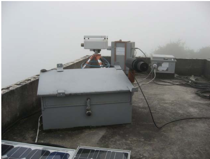
Fig. 5.30 – Photograph of the NOVAC site huayrapata, about 9 km northwest of the summit of Tungurahua Volcano. Here, three scanning DOAS instruments are installed on the roof of a small concrete structure. The NOVAC mark II instrument is mounted on a tripod between the other two scanners. In the foreground, the NOVAC mark I instrument is seen. It is installed in a large wooden box with the scanner protruding on the right side. In the back, a replica of the DOAS system applied on Soufrière Hills Volcano, Montserrat ( Edmonds et al. 2003a ) is set up. All instruments are powered by a land line buffered by two large car batteries located in the back right box. This housing also contains the radio modems used to send the spectral data to the Tungurahua Observatory located about 8km to the north.
