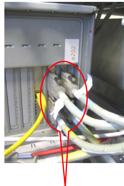
The SCI Cabling
