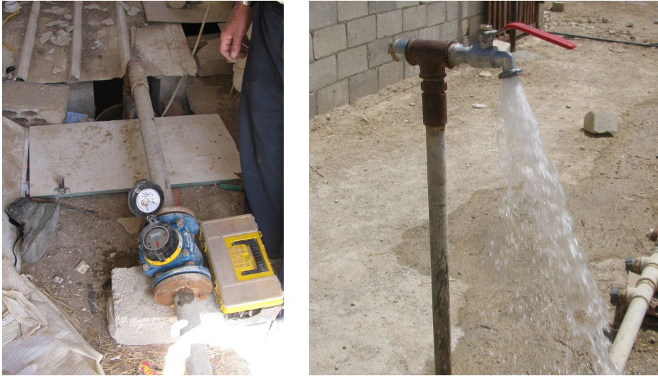
Figure A.3: Well head with flow meter and sampled tap of F3975
