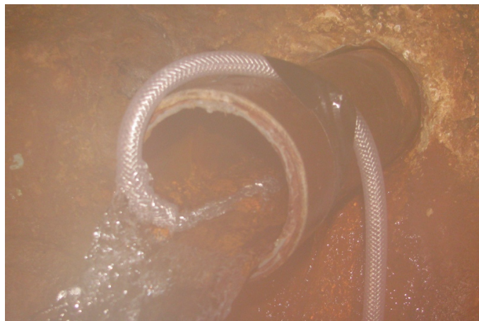
Figure A.9: The sampling tube was telescoped into the discharge pipe at Afra spring.
