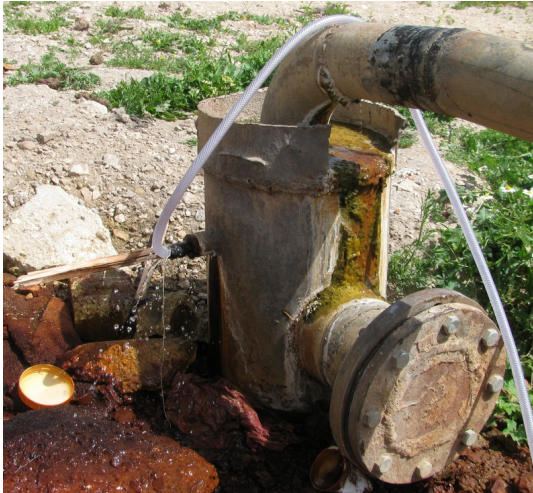
(a) Sampling hose connection at Manshiyeh 1
