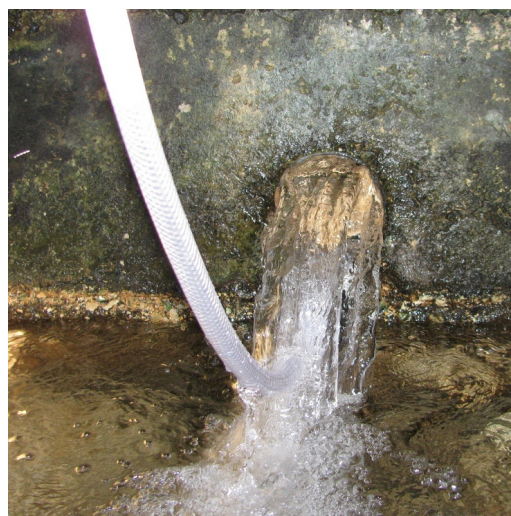
(b) Discharge pipe of Ibn Hammat I
