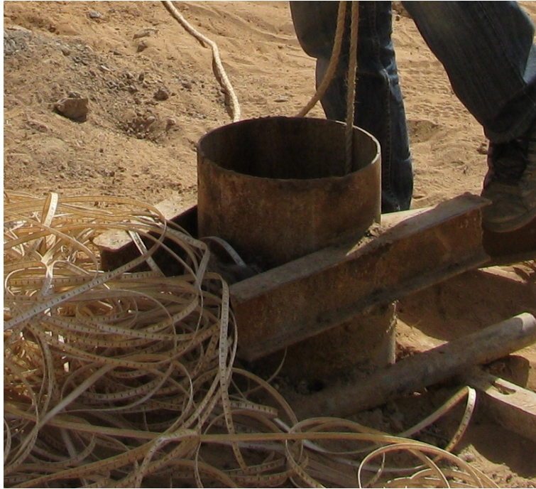
Figure A.5: Mohammeds well. There was no pump installed yet. Well F3960 was of the same type as this one.
