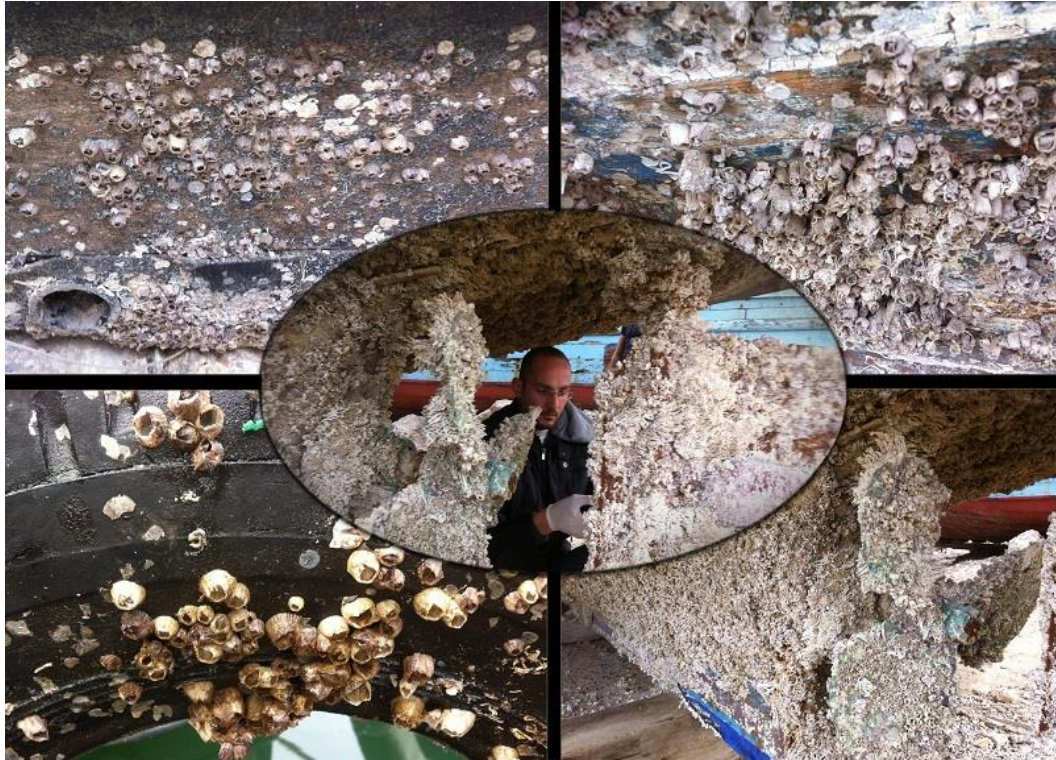
Figure 4: Consequences of barnacle invasion on boat hulls and pier structures. Images have been taken in Dekheila port, Alexandria, Egypt.
