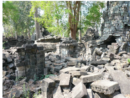
(b) The picture documents the state of deterioration inside the inner walls.
