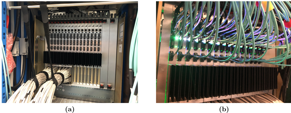
Figure 8.2. Bundles of LVDS cable insertion after the TREX installation (a), which connect to the CP and JEP systems. The optical fibre connection to the FEX and FELIX systems (b).
